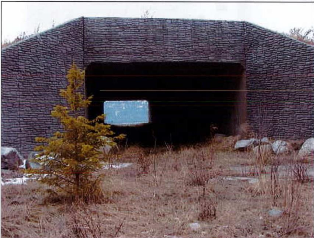
Figure 12. Wildlife underpass (box culvert) on the Copeland Project, Highway 95, north of Bonners Ferry, Idaho.
