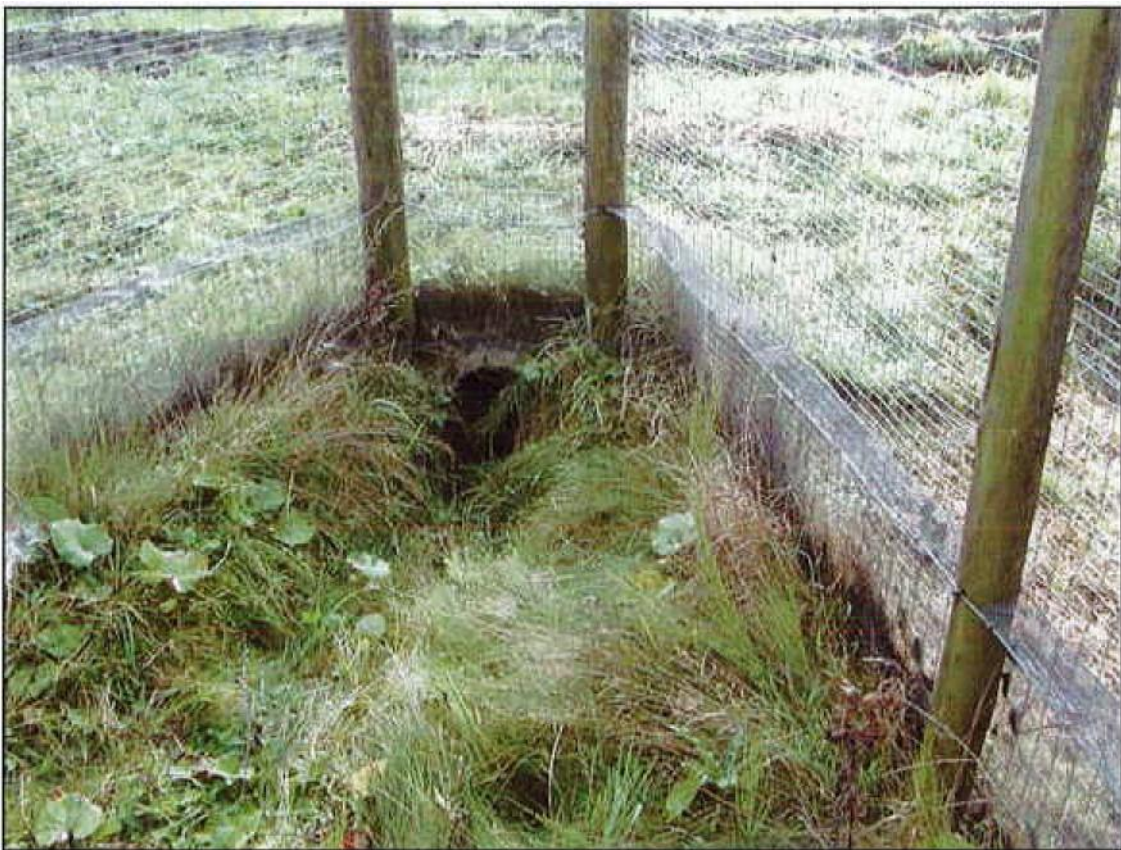
Figure 10. Small culvert in 'The Netherlands used for badger and other small animals. Note fencing.
